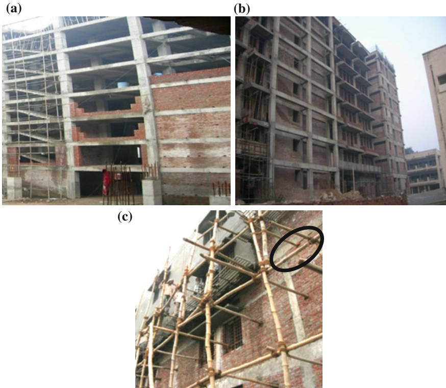
Fig. 3 Photographs showing typical construction sequence of an infilled frame building: a intermediate stage, b final stage of construction, c gap between infills and beam due to construction sequence of infilled frames
