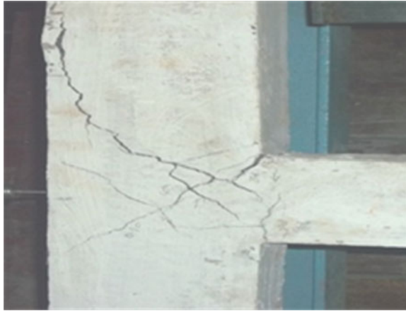
Fig. 8 Failure pattern of control specimen
