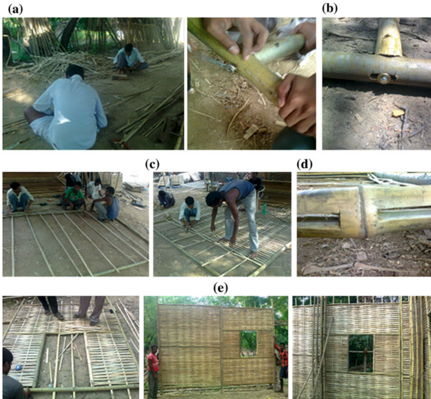
Fig. 3 Bamboo framed wall panel detailing. a Slivering of bamboo strips. b Assembly of bamboo frames with nut and bolts. c Making of bamboo panel using bamboo frames. d Grooves on intermediate bamboo frames. e Panel made with window opening and its installation
