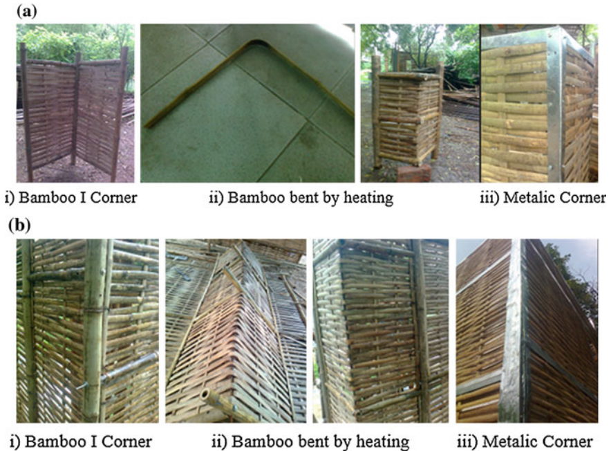
Fig. 5 Detailing of corner joints. a Development of modelled corner joints. b Different types of corner joints in real structure
