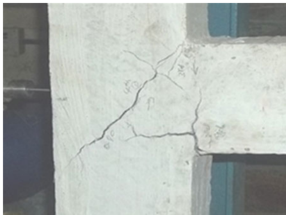
Fig. 7 Crack formation in joint region of control specimen
