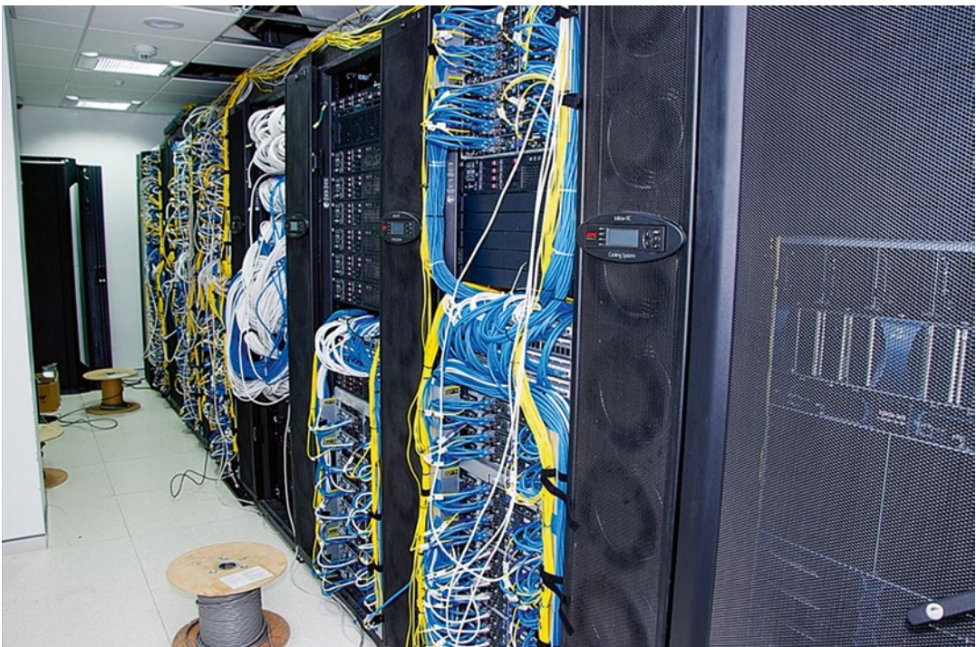
Fig. 5 High-performance computing facility at IASRI, New Delhi
