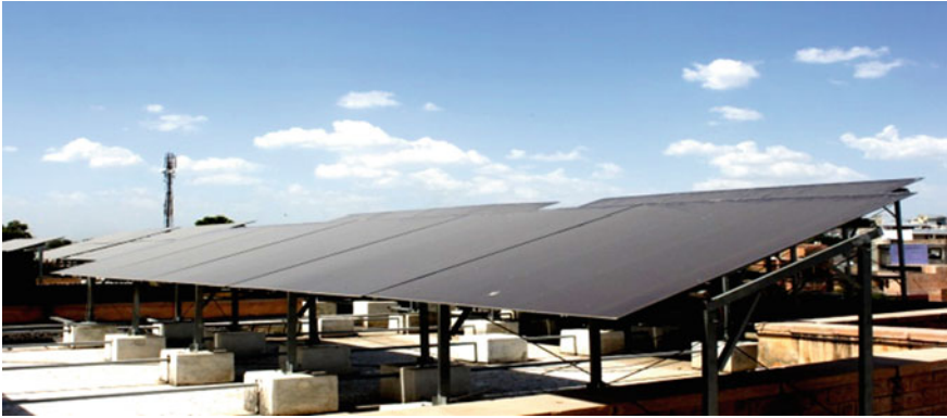
Fig. 5.3 43-kW A-Si-based solar PV system at rooftop
