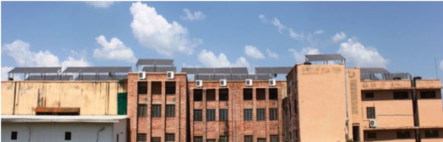
Fig. 5.2 Solar PV system at block-1 rooftop
