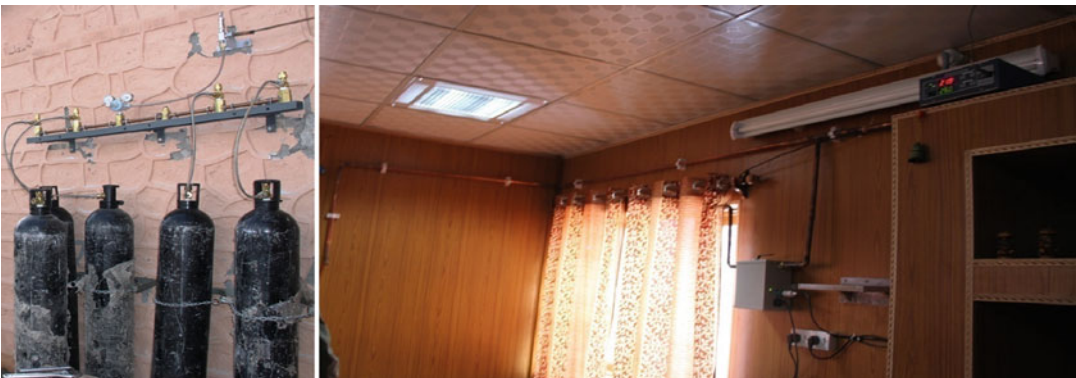
Fig. 11 Oxygen enrichment facility at Air Crew Resting Room, Leh Airport
