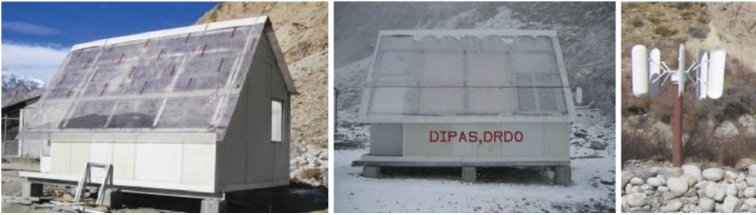
Fig. 1 Solar shelter along with vertical axis wind turbine installed at high altitude (Siachen Base Camp)
