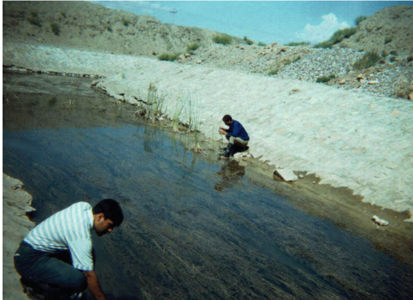
Fig. 10.4 Canal under construction in Hardwar (Uttarakhand state) for Tehri dam. It will remain a source of mosquito production and malarigenous conditions till the completion of the project. Thereafter, breeding will occupy seepage and agricultural fields
