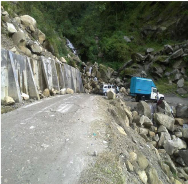
Fig. 4-3 Controlling measures around the Bagthang waterfalls in the form of buttressed retaining walls are no way effective in preventing landslides. The road has no culvert or x-drains. Boulders are constant threat to unwary travellers
