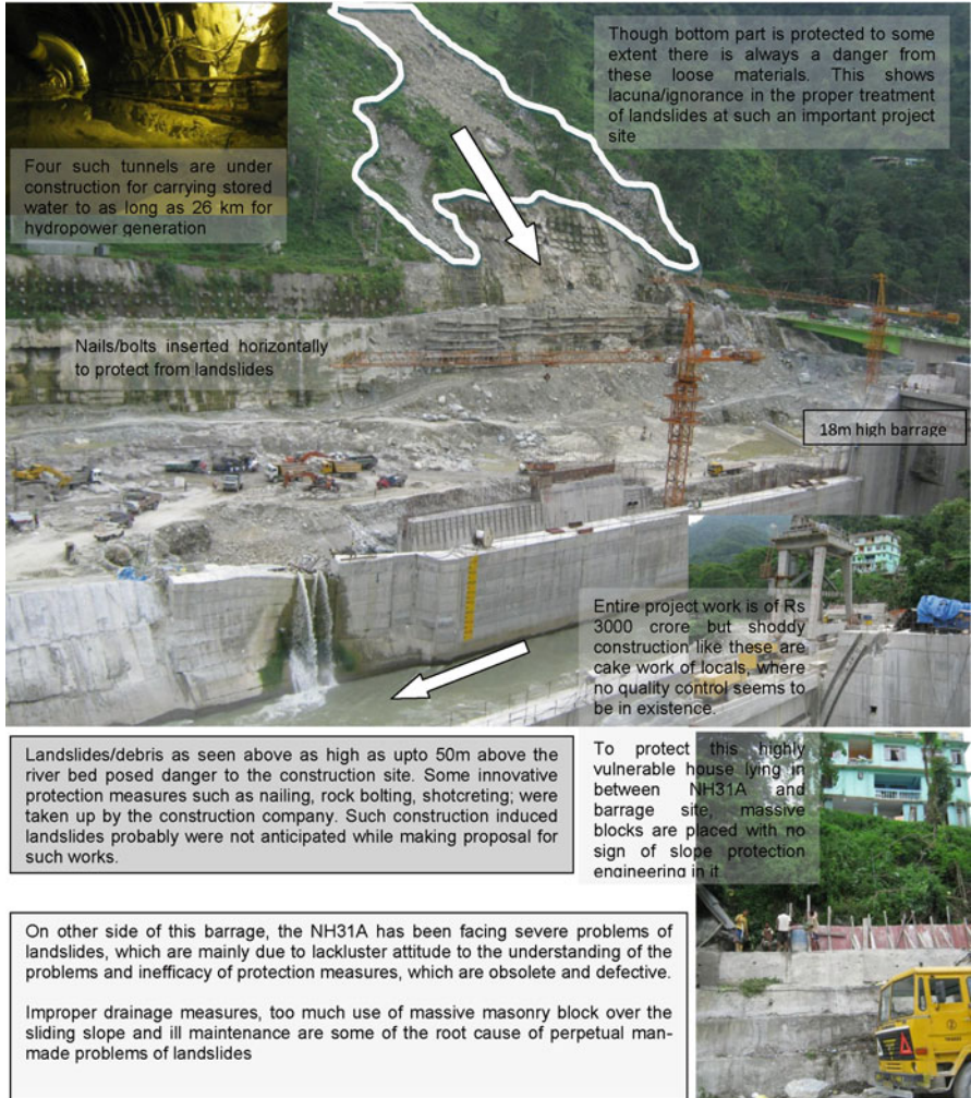
Fig. 3 Ongoing Barrage construction site at Sirwani, near Singtam, Sikkim state, along with 26 km tunnel for hydropower generation by Lanco Infratech Limited
