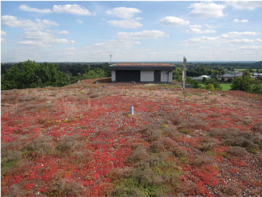
Fig. 10.8 Brown/biodiverse roof at Royal Holloway University of London (after Ishimatsu and Ito 2013)
