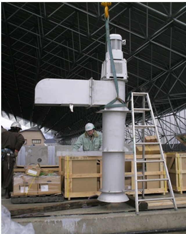
Fig. 7.12 Vertical pump with capacity of 250 tons water/hour
