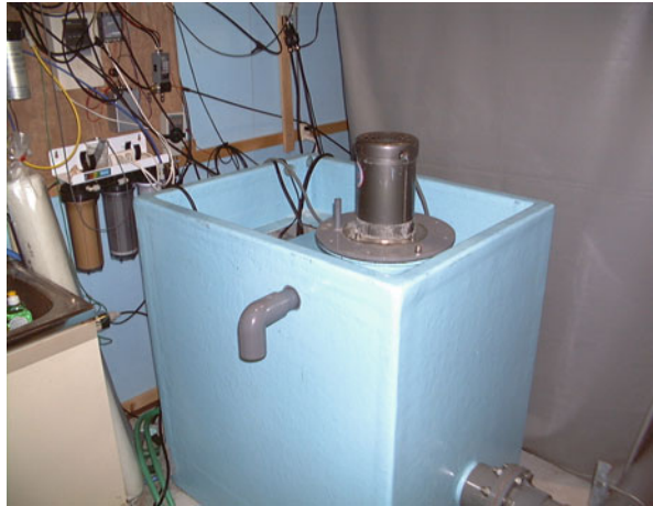
Fig. 4.5 Foam separation unit
