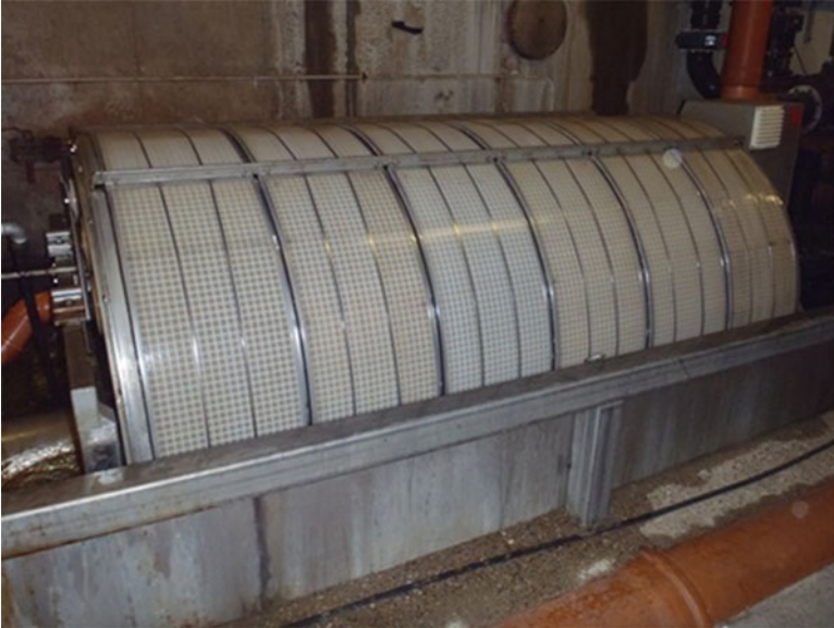
Fig. 2.4 Drum filter (Hydrotech, Inc.) using microscreen for physical treatment in CRAS
