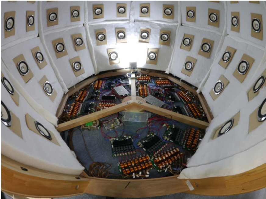
Fig. 2.6 Amplifiers and power supplies at the bottom of the cask
