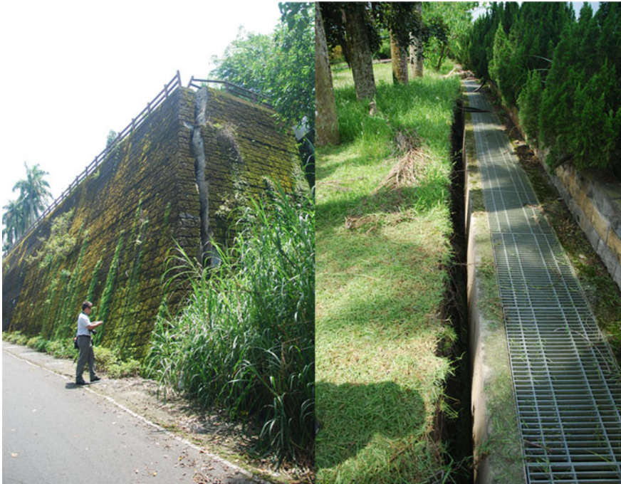
Fig. 4 Retaining wall failure case in Lugu Junior High School ( left the crack on the wing wall; right the separation of wall and backfill)
