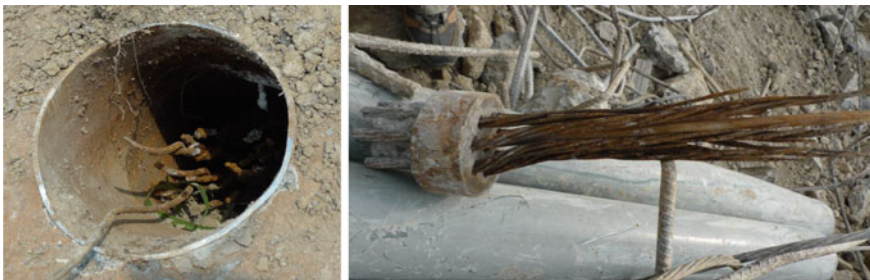
Fig. 2 Seriously corroded and broken steel strands found from at the landslide site
