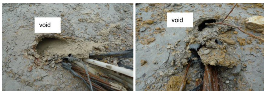
Fig. 4 UngROUTED free anchor end (inside and outside of plastic sheath) found from anchors left on sliding surface
