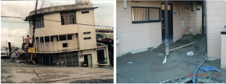
Fig. 1 Examples of liquefaction-damaged buildings: left tilted building after 1990 Luzon earthquake (Orense et al. 2011), right settlement of building due to liquefaction after 2011 earthquake of Japan
