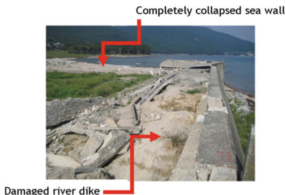
Fig. 1 State of damage of the Yoshihama dike
