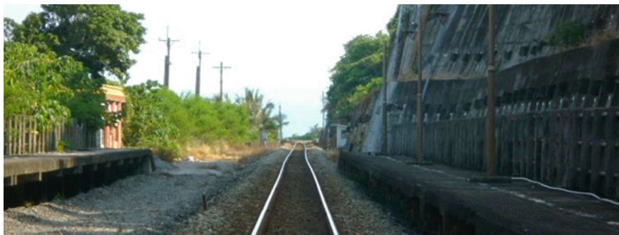
Fig. 3 Deformed rails next to a moving anchored slope
