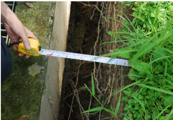
Fig. 6 Tape measurement of forward displacement on the top of the retaining wall
