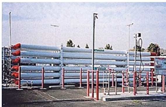
Fig. 4.44 Simple hydrogen dispenser
