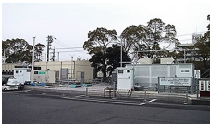
Fig. 4.46 Takamatsu H 2 station
