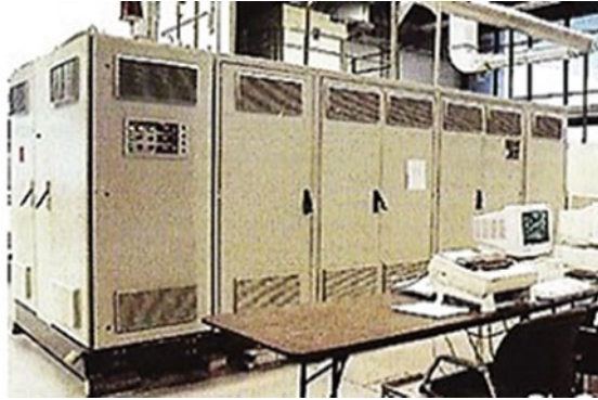
Fig. 5.23 WH 25 kW solid oxide fuel cell (SOFC) at Osaka Gas. Source Osaka Gas Co.
