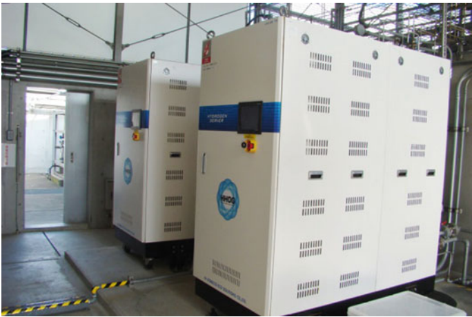
Fig. 2.11 Polymer electrolyte fuel cell (PEFC)-type water electrolysis system (inside the hydrogen filling station at Kyushu University)
