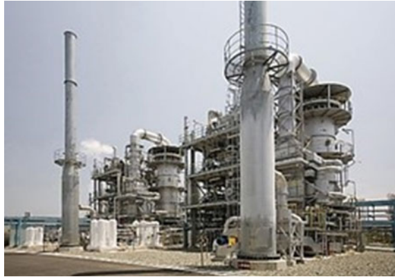
Fig. 4.10 2700 Nm 3 /h natural gas reformer (Source HydroEdge)
