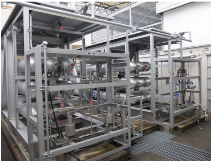
Fig. 2.12 Hydrogen tanks for high-pressure hydrogen storage (inside the hydrogen filling station at Kyushu University)
