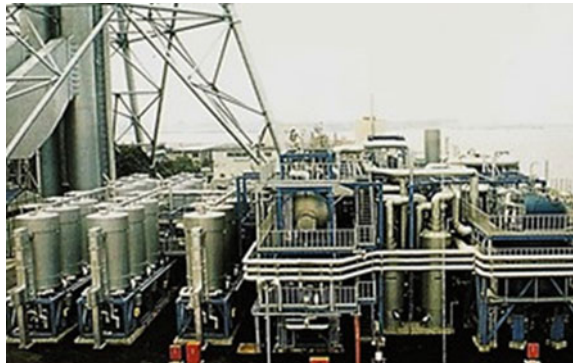
Fig. 5.8 World's largest 11 MW PAFC. Source Toshiba FC Power Systems
