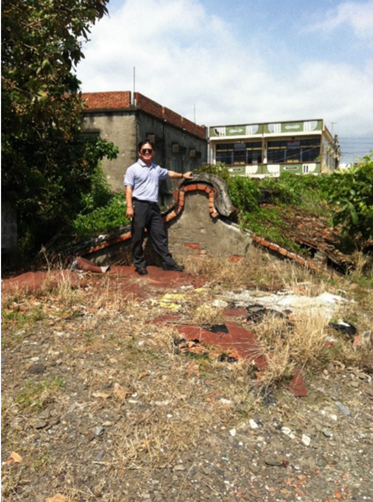
Fig. 7.3 A traditional house which has been consumed by land subsidence (Source: taken by author, Jia-tung Township, Pingtung County, July 2014)
