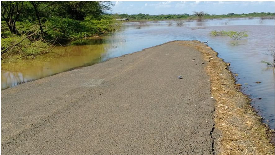
Fig. 12.10 Floodwaters cut off the road infrastructure around Lake Bogoria (December 2013)
