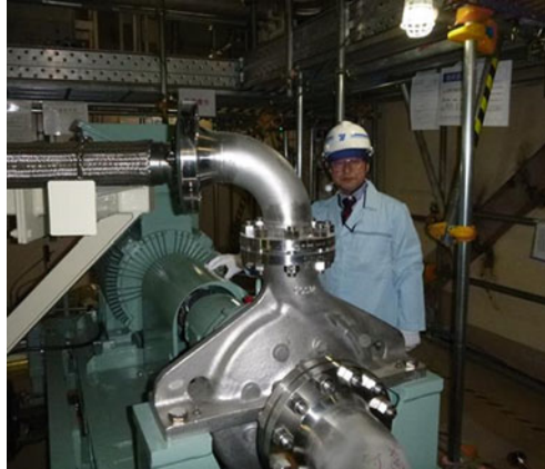
Fig. 37 Water injection pump
