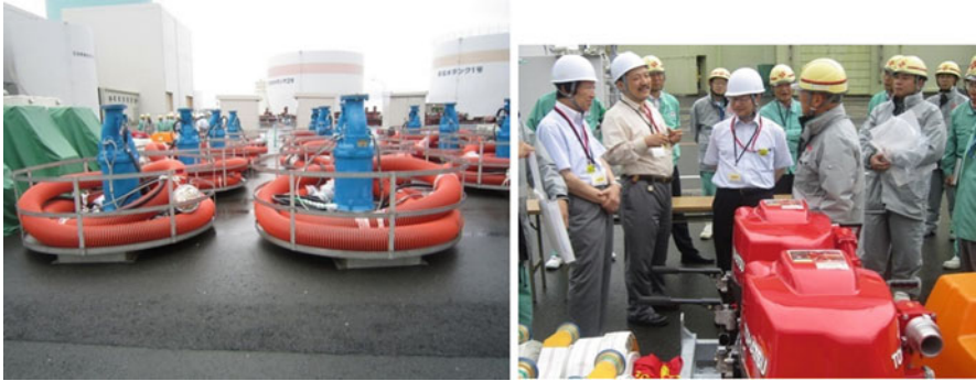
Fig. 39 Mobile pumps deployed in Ikata NPS [14]
