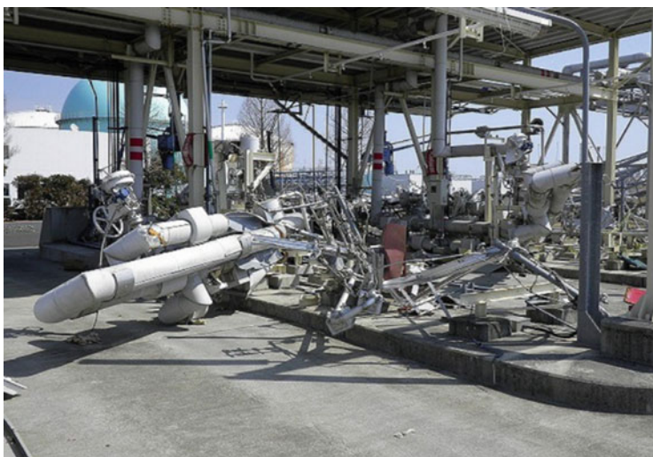
Fig. 1 Damage to LNG terminal from tsunami caused by 2011 Tohoku earthquake off the Pacific coast (shipping facilities for LNG tank truck) [3]
