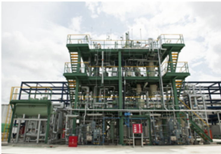
Fig. 1 Demonstration plant of SPERA Hydrogen™ (2013, Kawasaki). Capacity of 50 Nm 3 H 2 /h for TOL hydrogenation and MCH dehydrogenation would be enlarged upon demand requests
