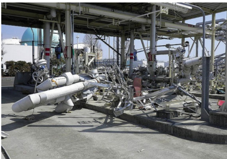
Fig. 1 Damage to LNG terminal from tsunami caused by 2011 Tohoku earthquake off the Pacific coast (shipping facilities for LNG tank truck) [3]
