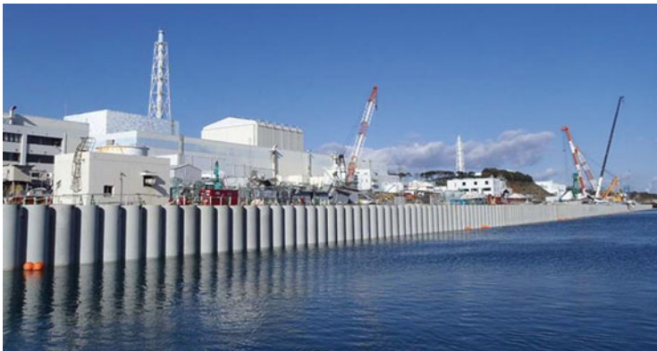
Fig. 56 Impermeable wall to prevent contaminated water flowing into the sea [18, 19]
