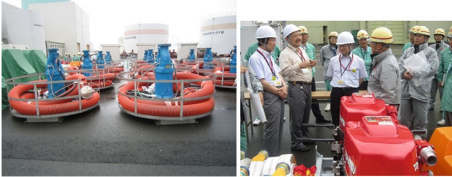
Fig. 39 Mobile pumps deployed in Ikata NPS [14]
