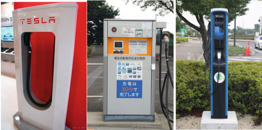
Fig. 8 Examples of charging equipment for BEVs/PHEVs (left: TESLA supercharger, middle: quick charger, Right: 200-V normal charger)
