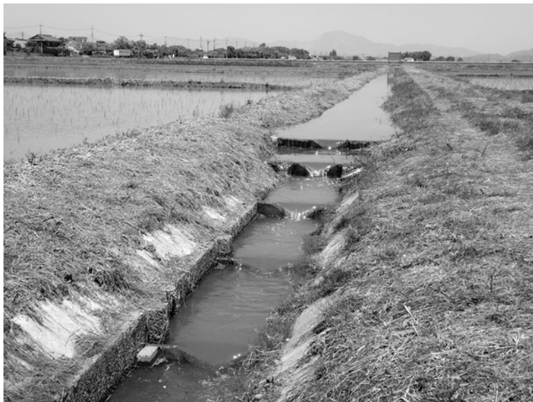
Fig. 10.3 A fish-ladder cascade installed in a drainage canal as part of the Sakana-no-yurikago-suiden fish nursery program in rice fields (Photo by Shigefumi Kanao)
