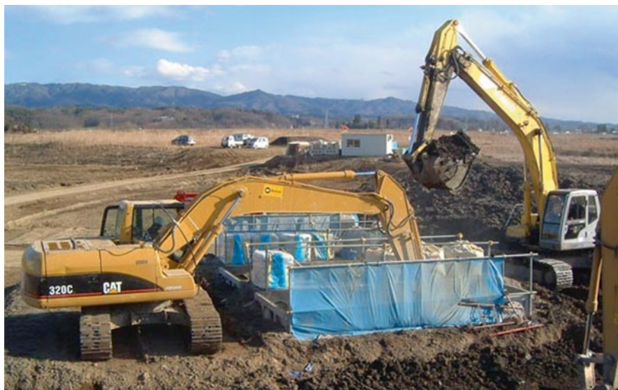
Fig. 10.8 Construction of river bank in Hamao area, Fukushima Prefecture. The backhoe on the right side of the photo is putting in high moisture content mud into the pits; the left backhoe with mixing attachment is mixing with paper and materials and providing agitation
