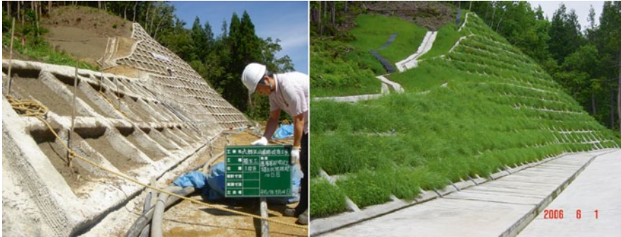
Fig. 10.13 Spray construction ( left ) and greening of the face after growth of vegetation ( right ): National Highway 13
