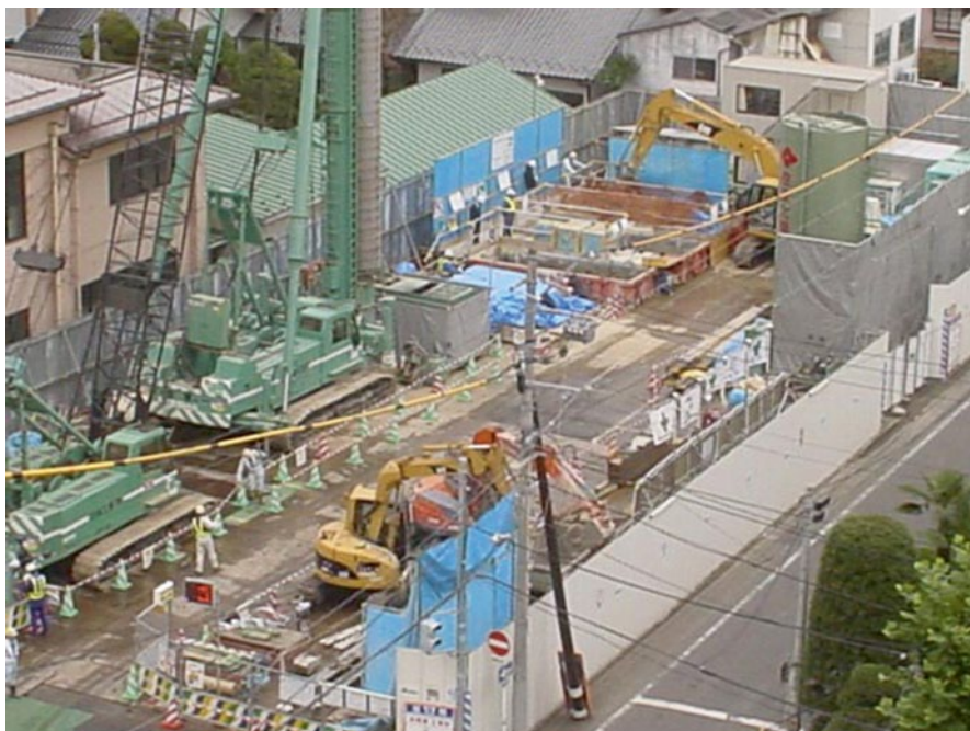
Fig. 10.9 Construction of public utility conduit in Sendai (Miyagi Prefecture). Unlike Fig. 10.8, the construction site is located close to the center of town, so there is only limited work area requiring heavy equipment to be efficiently located and uncluttered. Upper right half of the photograph shows the ‘Bon terrain’ method location with loading and mixing underway
