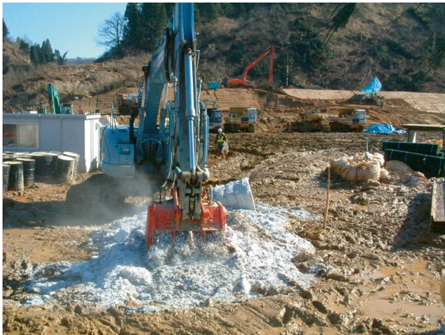
Fig. 10.10 Urgent countermeasures construction to respond to sediment-related disasters. Paper shredder residue mixed with soft soil; the rapid stabilization helps speed up the restoration work
