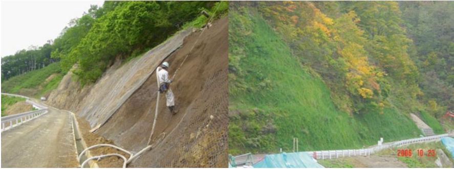
Fig. 10.14 Spray construction ( left ) and greening of the face after growth of vegetation ( right ): Okura, Mogami, Yamagata Prefecture
