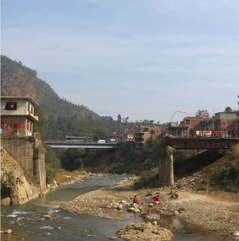
Fig. 4.6 Collapse of bridge over Malekhu River in central Nepal by the impact of huge amount of debris brought by 1993 central Nepal cloudburst
