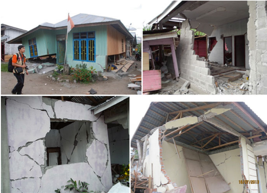
Fig. 17.8 Typical damaged houses (mixed masonry and timber house, cement brick material, diagonal cracks, collapse of adjoining walls)
