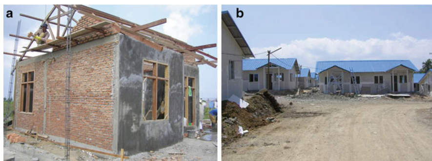
Fig. 17.1 (a) Type 36 houses under construction by BRR. (b) Houses with imported materials
