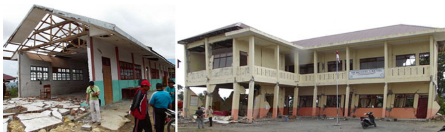
Fig. 17.10 Damaged school buildings
