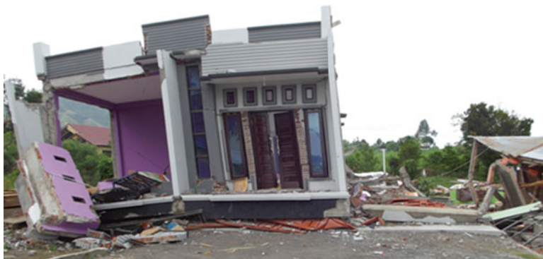
Fig. 17.9 Soft story failure of two storied house
