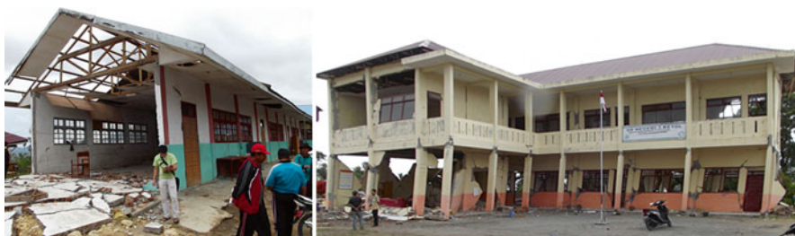
Fig. 17.10 Damaged school buildings
