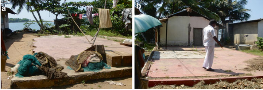
Fig. 28.3 Previous community of eco-village people. (a) Damaged house by tsunami of Eco-villagers at Kartala South. (b) Damaged house in previous land and house owner
