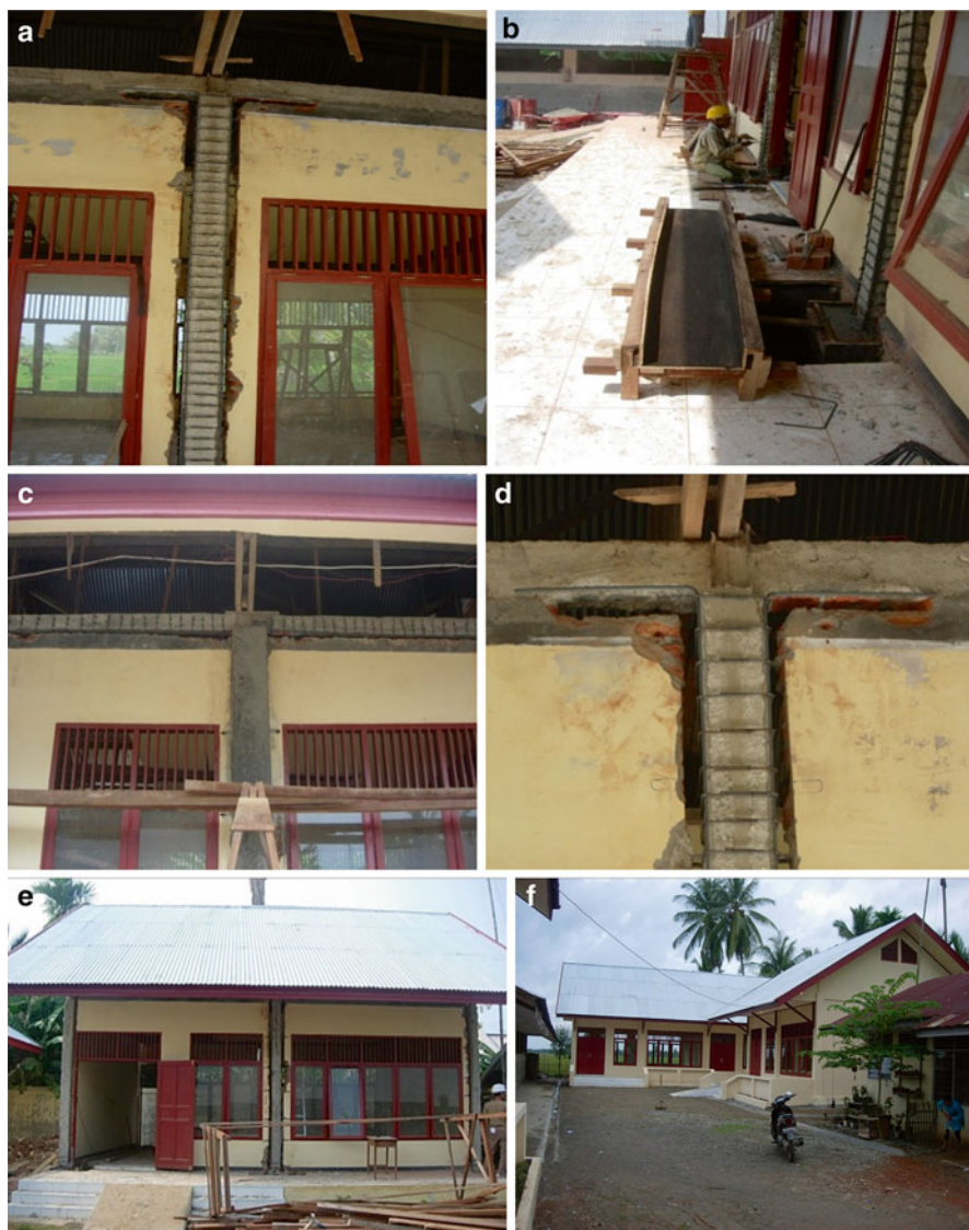
Fig. 16.14 A building during retrofitting and after completion. (a) Retrofitting of column. (b) Retrofitting of foundation and form work for column. (c) Retrofitting of beam. (d) Joint between column and beam. (e) Building on retrofitting process. (f) Building after retrofitting
