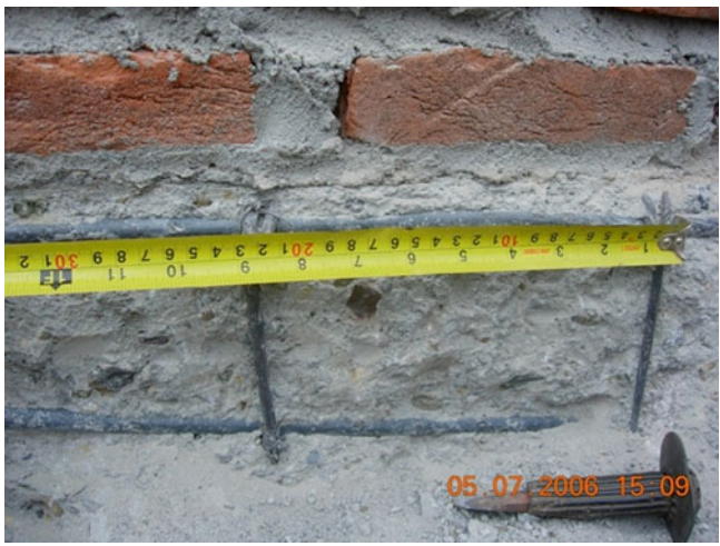
Fig. 16.5 Poor quality reinforcement detail
