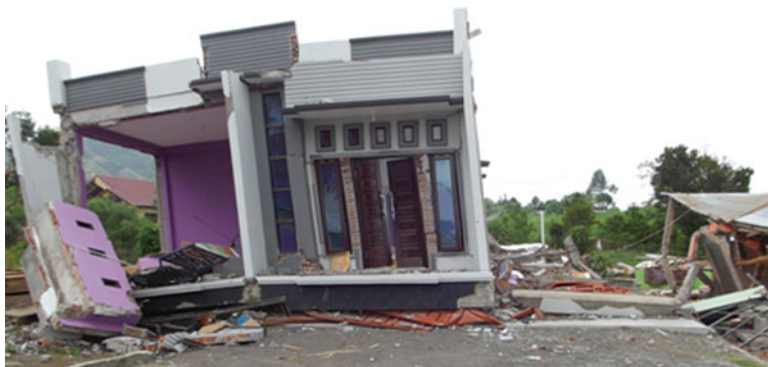
Fig. 17.9 Soft story failure of two storied house
