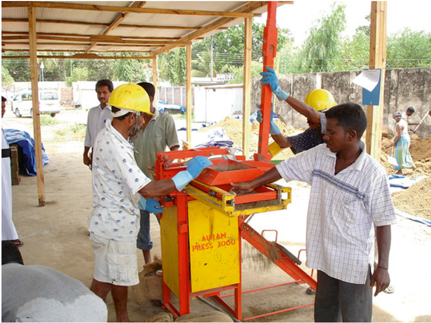
Fig. 27.6 Production of compressed soil-cement blocks for building walls in Caritas shelter projects created livelihood opportunities ( Photo: courtesy of I. Anda )
