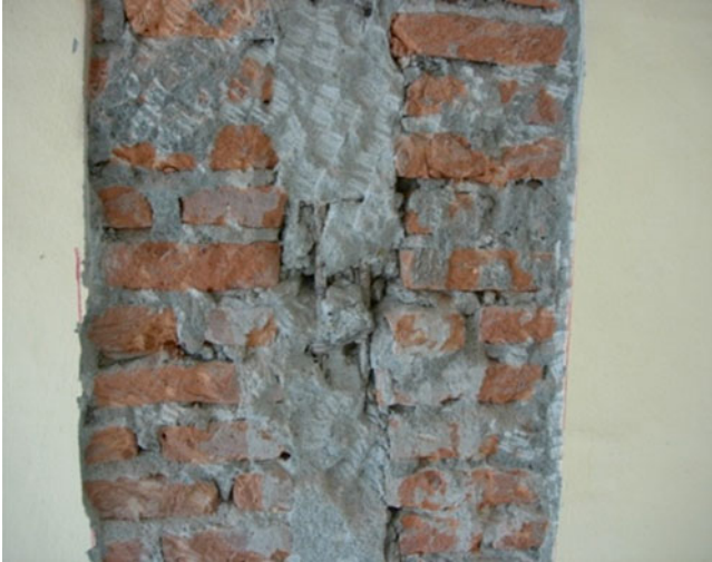
Fig. 16.3 Poor quality concrete work
