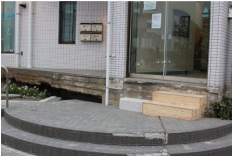
Fig. 10.9 Ground sinkage around a pile foundation building
