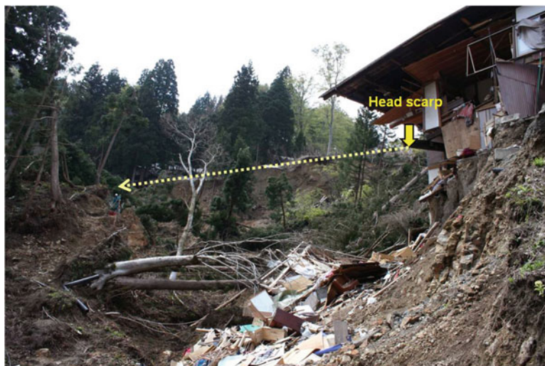
Fig. 11.10 Head scarp and landslide moving body remaining on a hillock
