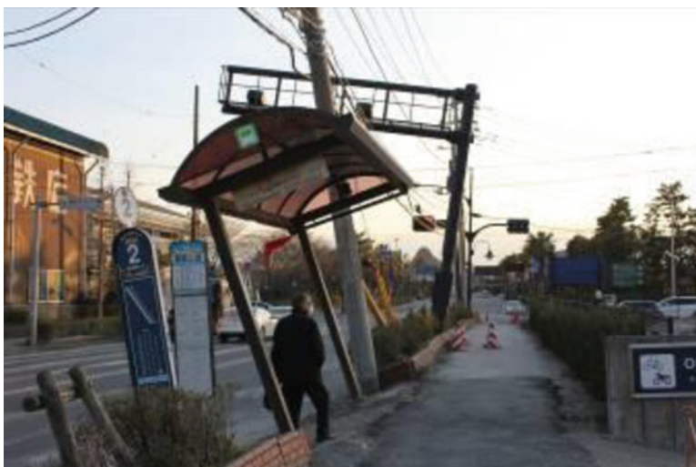
Fig. 10.7 Damage to a sidewalk
