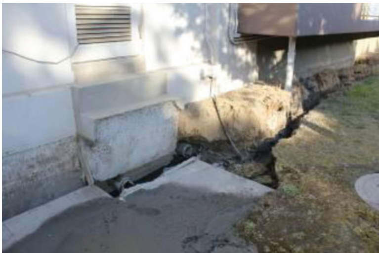
Fig. 10.10 Severed lifeline at the border between the building and the ground
