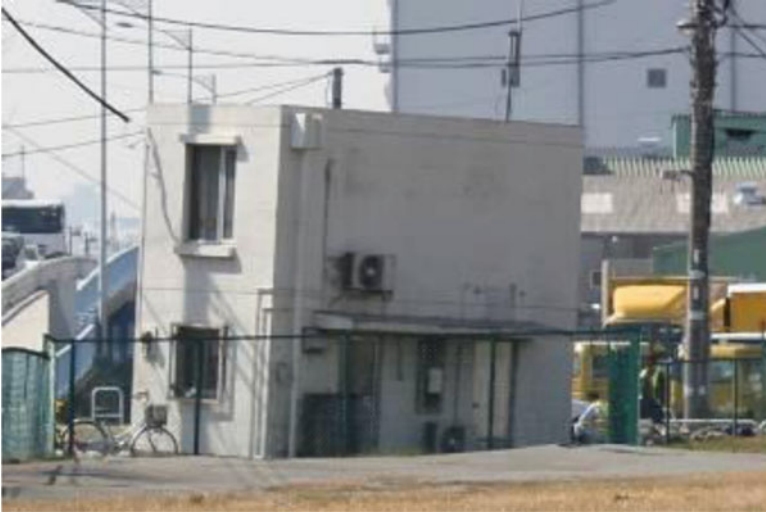
Fig. 10.25 Sunken and tilted two-storey reinforced concrete building
