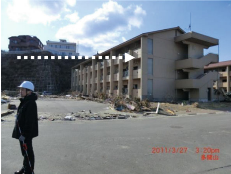
Fig. 4.12 Survived concrete-reinforced apartment building at the coast
