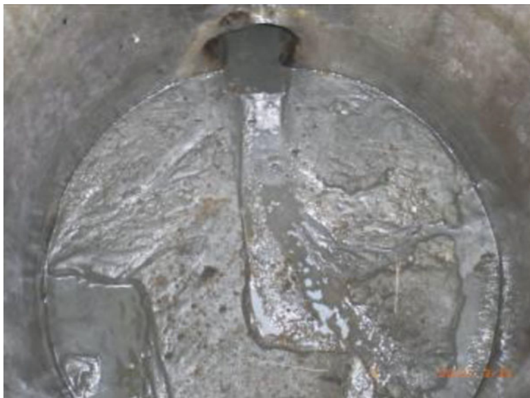
Fig. 10.14 Sand flown into a manhole (photo by Mr. Y. Kamiya)
