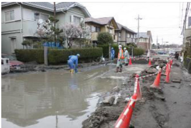
Fig. 10.15 Sediment erosion due to a ruptured water pipe
