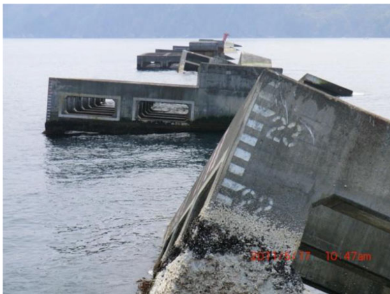
Fig. 4.15 Kamaishi breakwater after tsunami event
