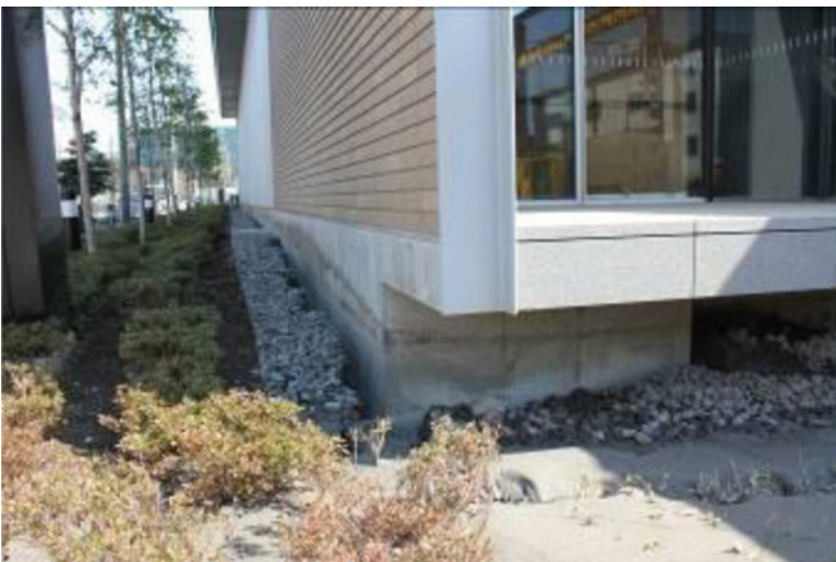
Fig. 10.26 Ground sinkage around a pile foundation building
