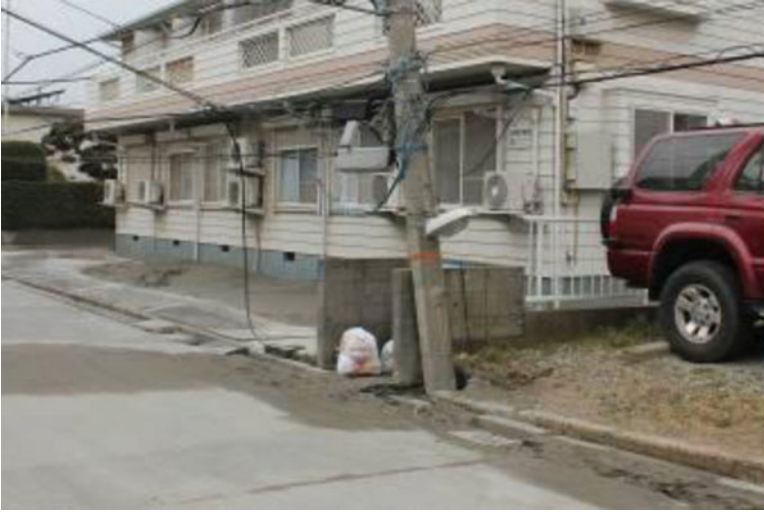
Fig. 10.12 Sinkage at a utility pole
