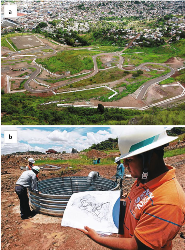
Fig. 9.7 Countermeasures carried out by JICA to reduce the landslide risk in El Berrinche Hill. a Channels that transport surface water are shown. b One of the drainage wells with intake pipes at different depths to collect groundwater is shown. Both figures were taken from El Heraldo newspaper and were published on April 7, 2014
