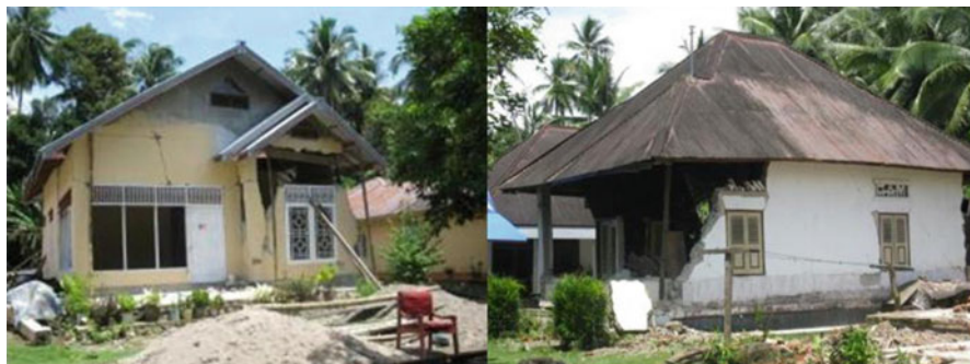
Fig. 11.6 Earthquake damaged houses in Padang Pariaman, West Sumatra. The house on the left was rehabilitated by the owner with own fund, while the one on the right waited for the disbursement of government aid ( source : Field Observation in Padang Pariaman 2006)
