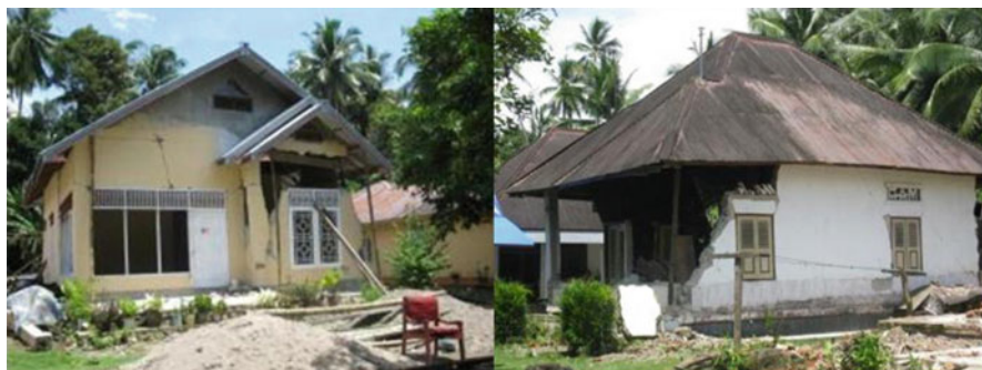
Fig. 11.6 Earthquake damaged houses in Padang Pariaman, West Sumatra. The house on the left was rehabilitated by the owner with own fund, while the one on the right waited for the disbursement of government aid ( source : Field Observation in Padang Pariaman 2006)
