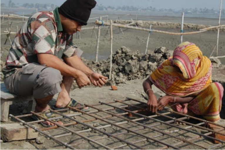
Fig. 13.6 A student volunteer and local lady tying reinforcement bars (photo: Hasibul Kabir)
