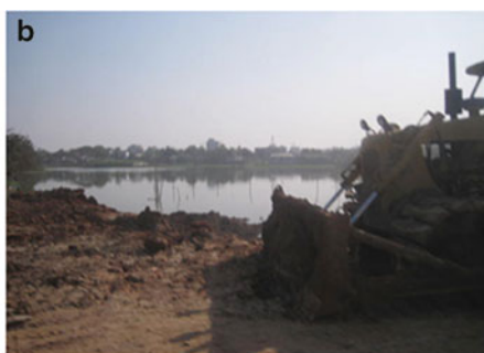
b Filling of water bodies for Housing Project (Basundhara City Project, Zone No. 9)
