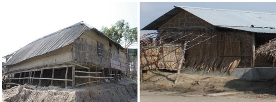
Fig. 10.2 Increasing plinth level of house ( left ) and concrete plinth ( right ) using locally available materials
