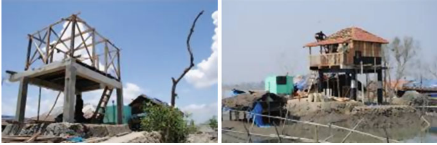
Fig. 17.6 Individual house construction in progress for the climate resilient habitat project in Satkhira. Source: Khandoker Hasibul Kabir, Department of Architecture, BRAC University
