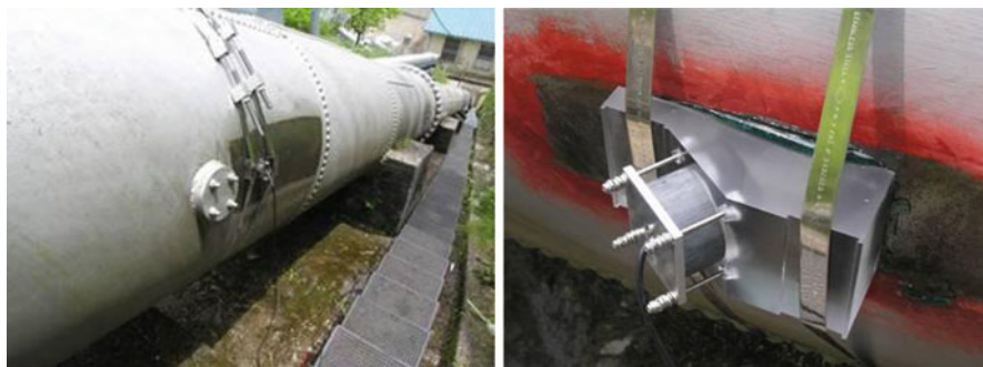
Fig. 5.83 Ultrasonic transducer and wedge installed on the surface of a steel penstock (reprinted from [111] with permission from Elsevier)
