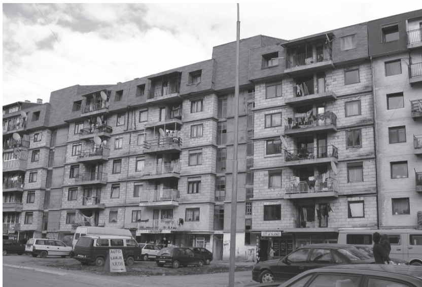
Fig. 7.2 Multi-apartment housing built in the early 1990s in Pristina with visible signs of deterioration
