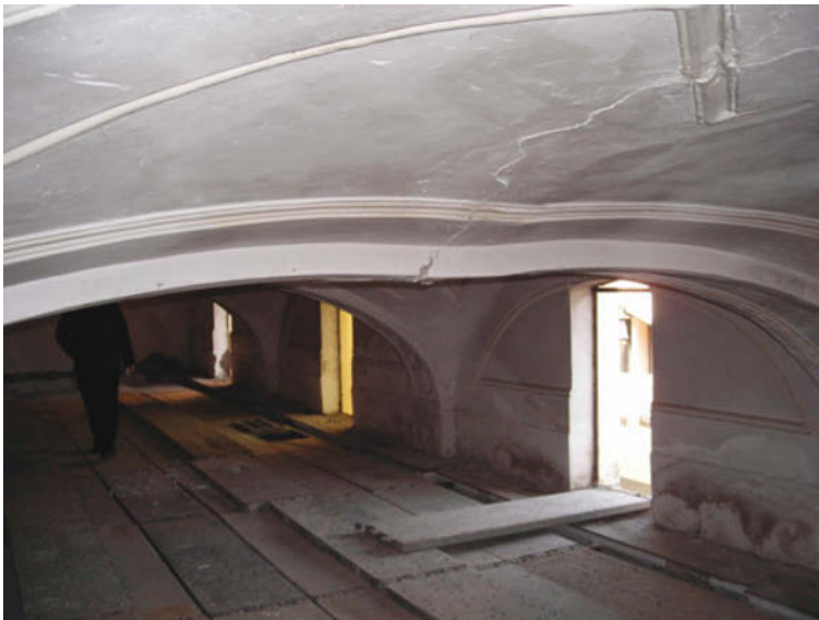
Figure 6. Incipient failure of a shallow cross vault due to excessive spread of the abutments (aisle vaults of a XVI century chapel in Nocera Inferiore (SA), Italy). Courtesy of Enrico Sicignano.
