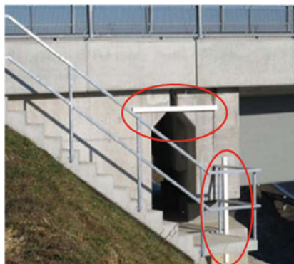
Fig. 9 View of the sensor attached to the deck of the bridge
