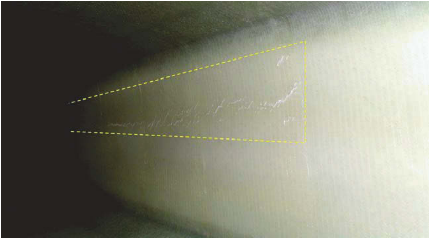
Figure 34. Image from inside the blade showing damage
