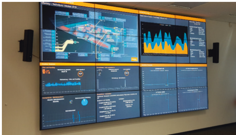
Fig. 7.9 Monitoring system at the Nerve Centre of the Open Hybrid LabFactory
