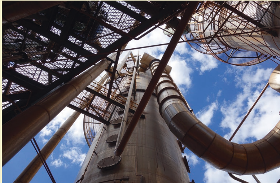
Partial view of a distillation column for bioethanol in Brazil (© Usina Nova Gália Ltda.)
