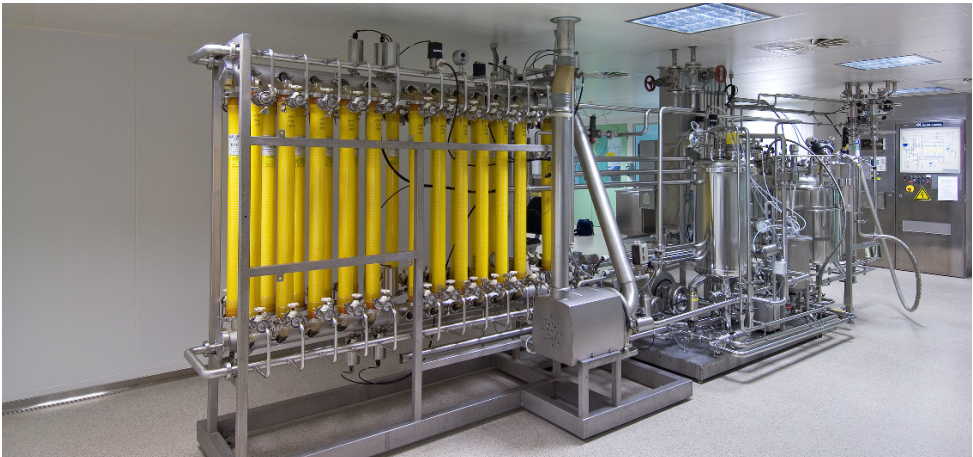
Fig. 14b. Ultrafiltration facility
