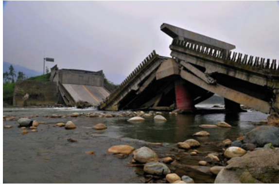
Fig. 1.16 Bridge collapse in the Wenchuan earthquake
