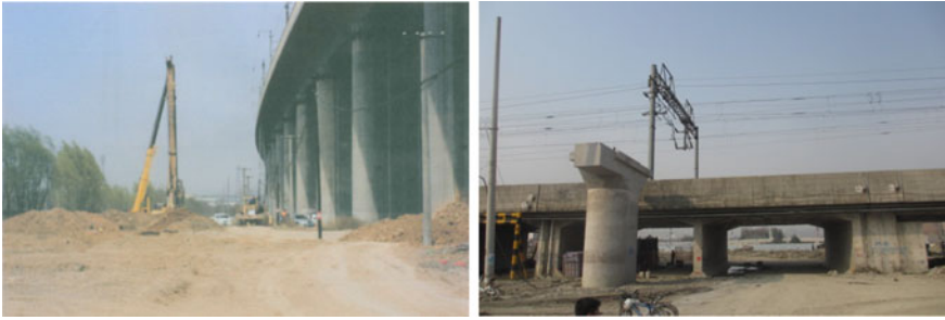
Fig. 9.3 Construction of a new bridge parallel to the existing railway (Taken on Datong-Xi'an HSR line construction site)
