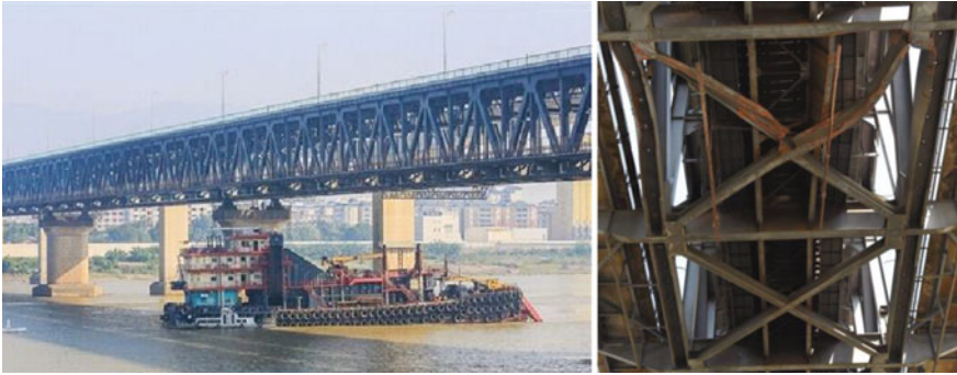
Fig. 1.21 Ship collision induced damage of Zhaoqing Bridge on Xijiang River (ifeng 2015)
