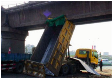
(a) A railway bridge hit by a dumper in Xinjiang (v.ku6, 2008)
