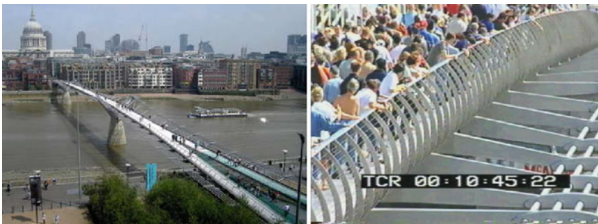
Fig. 1.28 London Millennium Bridge was closed due to crowd-induced vibration
