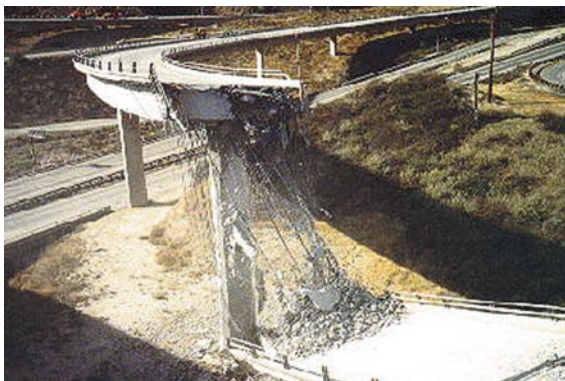
Fig. 1.15 Bridge collapse in the Northridge earthquake (Cooper et al. 1994)
