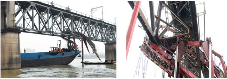
Fig. 1.22 Ship collision induced damage of Xiangtan Bridge on Xiangjiang River (hnxttv 2016)
