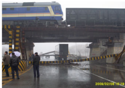
(b) A railway bridge hit by container in Heze
