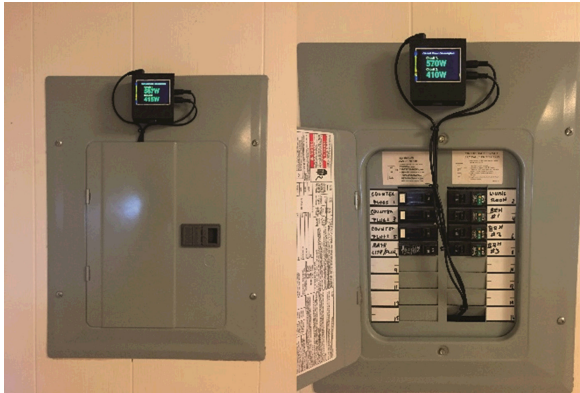
Fig. 3. A SPM meter is installed in the circuit breaker box of a home taking part in the pilot project.
