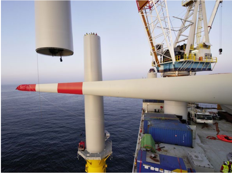
■ Fig. 11.3 A tower segment being raised from the installation vessel and onto the segment already in place where the service technicians are ready and waiting. Part of the 56.5-metre-long rotor blade can be seen in the foreground. © Adwen/Jan Oelker
