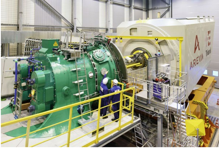
■ Fig. 11.5 Inside view of the Adwen test stand. © Adwen/Jan Oelker
