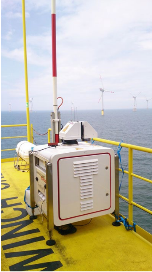
Fig. 13.1 Long-range lidar on the Alpha Ventus transformer platform. © ForWind – University of Oldenburg
