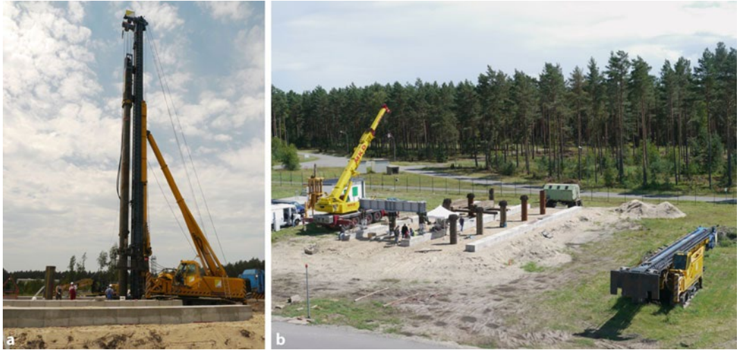
Fig. 7.2 Horstwalde test field. a Driving a pile, b View of the test field with ten piles (length 20 m, diameter 0.7 m). © BAM
