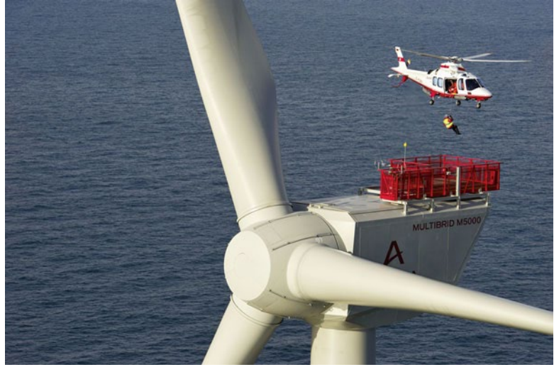
■ Fig. 11.7 A technician is lowered onto the winch platform for a service assignment. © Adwen/Jan Oelker
