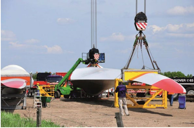
■ Fig. 9.3 The prototype of the rotor blade is prepared for installation. © Senvion GmbH 2015
