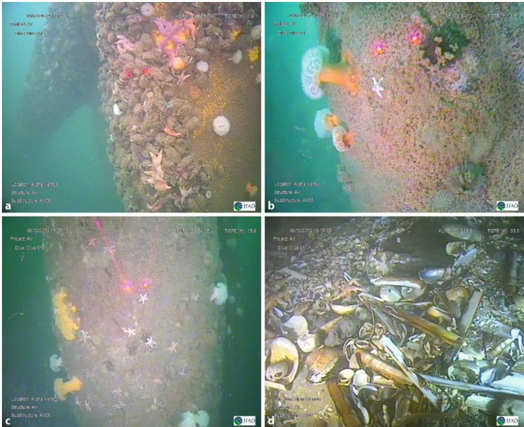
■ Fig. 5.3 Marine growth at different depths on the foundations of turbine AV6 and on the seabed. a –1.9 m, b –8.6 m, c –15.8 m, d –33.0 m (seabed). © IfAO
