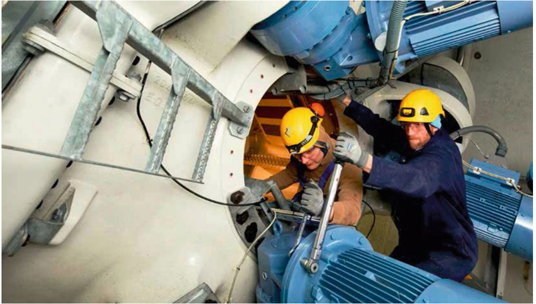
■ Fig. 8.2 Installation of the pitch mechanisms in the hub of a Senvion offshore wind turbine. © Senvion GmbH 2015
