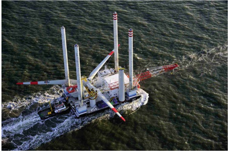
Fig. 1.2 July 2009: Transporting the first offshore wind turbine to the Alpha Ventus construction site. © DOTI/Alpha Ventus (Photographer: Mathias Ibeler)
