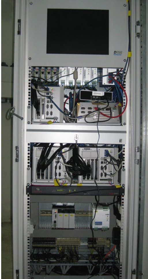
■ Fig. 3.2 Control box for research measuring equipment in an offshore wind turbine. © UL International (DEWI)
