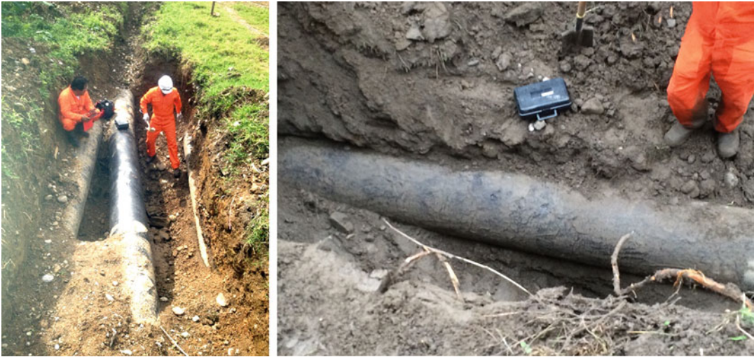
Corrosion, Fig. 8 Underground pipeline corrosion (original)
