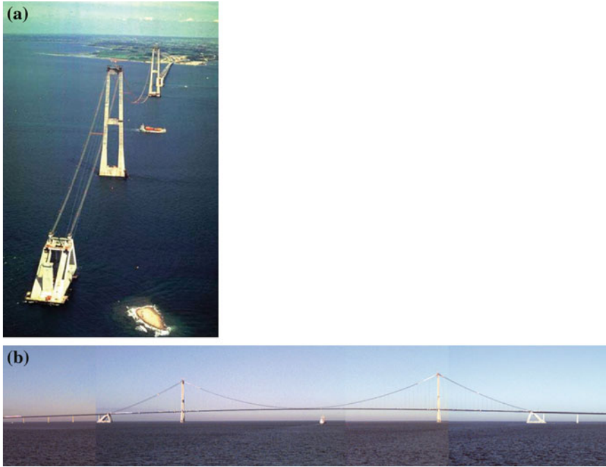
Fig. 14 Aerial photos of the Great Belt Bridge, Denmark: a during the construction and b after completion (after Lee et al. 2006)
