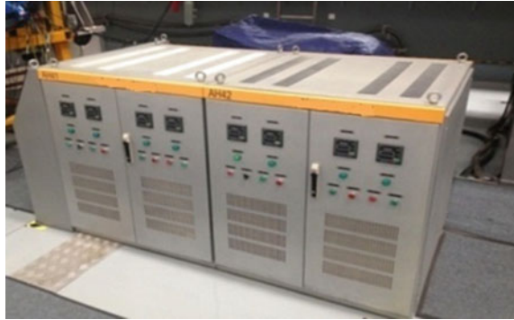
Fig. 49.6 The control cabinet of electric axis system
