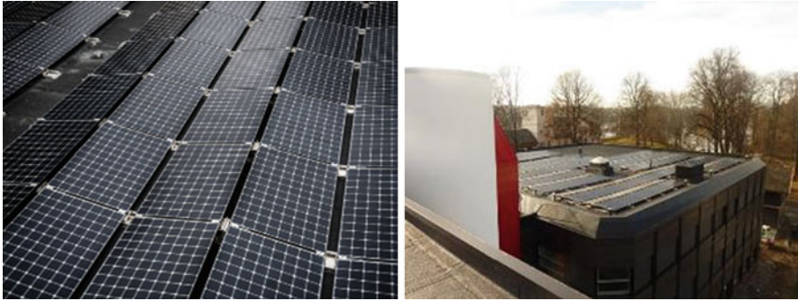
Fig. 9 Photos showing the placement of the PV panels on the roof. Photos: Skanska
