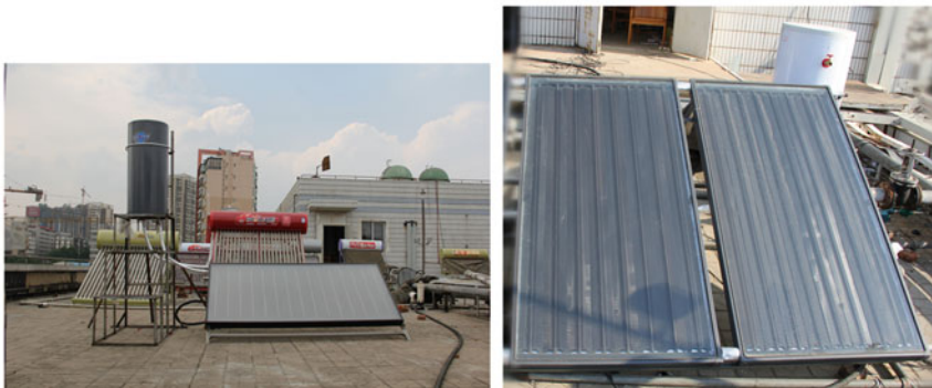
Fig. 1 Cross section of a typical flat-plate solar collector ( up ), photo of collectors ( down )
