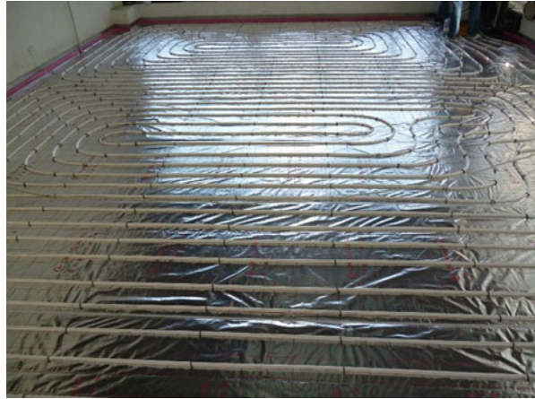
Fig. 39 floor-heating coils used in the test room
