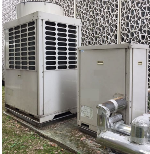
Fig. 24 Outdoor unit and expansion tank
