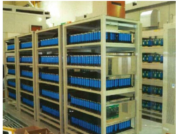
Fig. 16.41 Large EC storage system used to improve power quality. This system delivers 2 MW for 1.5 s (courtesy of Nippon Chemi-Con Corporation)
