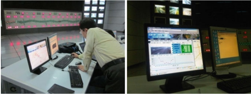
Fig. 31.5 Demonstration application of the comprehensive analysis and early warning expressway weather information system
