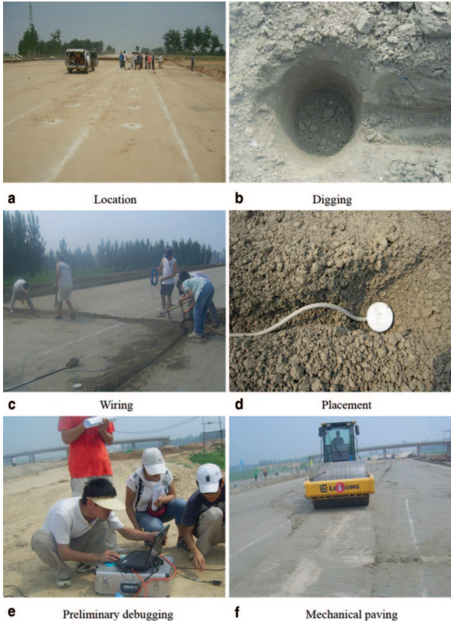
Fig. 10.4 Sensor layout process. a Location. b Digging. c Wiring. d Placement. e Preliminary debugging. f Mechanical paving
