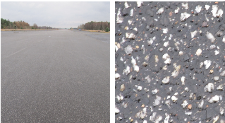
Fig. 3. View of the investigated bituminous pavement (left photo) and its structure (right photo) [own study]
