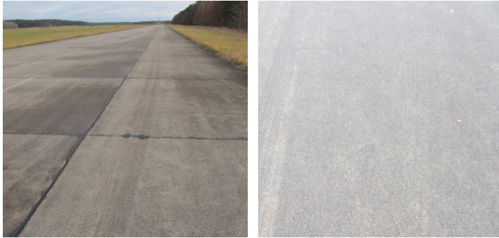
Fig. 2. View of the investigated concrete pavement (left photo) and its structure (right photo) [own study]
