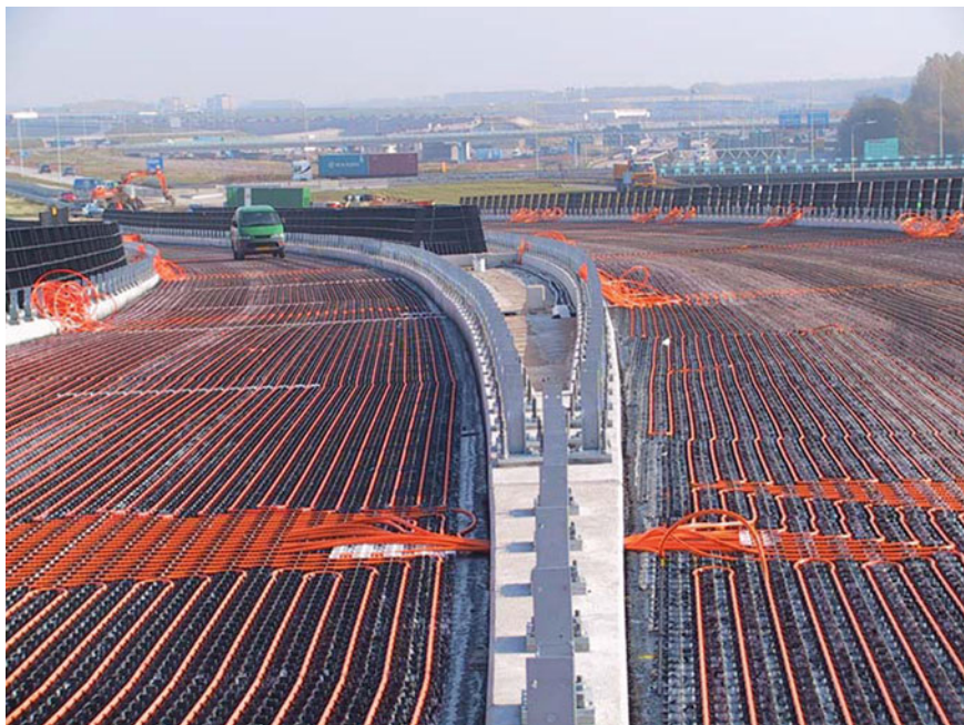
Fig. 18.8 Asphalt solar collector system under construction on a bridge in Rotterdam (de Bondt 2003)
