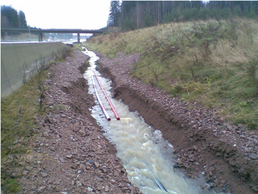
Fig. 4.6 Excessive run-off/seepage eroding the top of a drain following heavy rainfall (courtesy of Antero Nousiainen)
